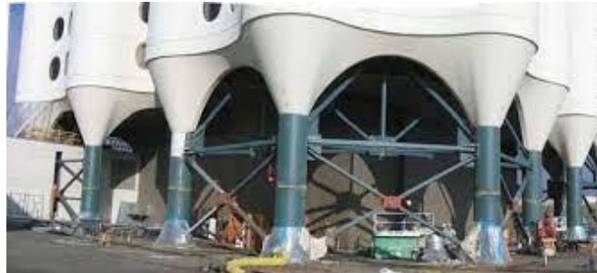
Figure 5 Saint Joseph Hospital, Patient Towers, Seattle, 40' Soft Story, Retrofitted with X-Brace PFDS
